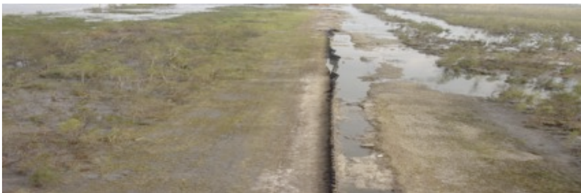
Figure 13. Levee Damage after Hurricane Katrina
