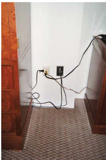
Visible cords in guestroom.
