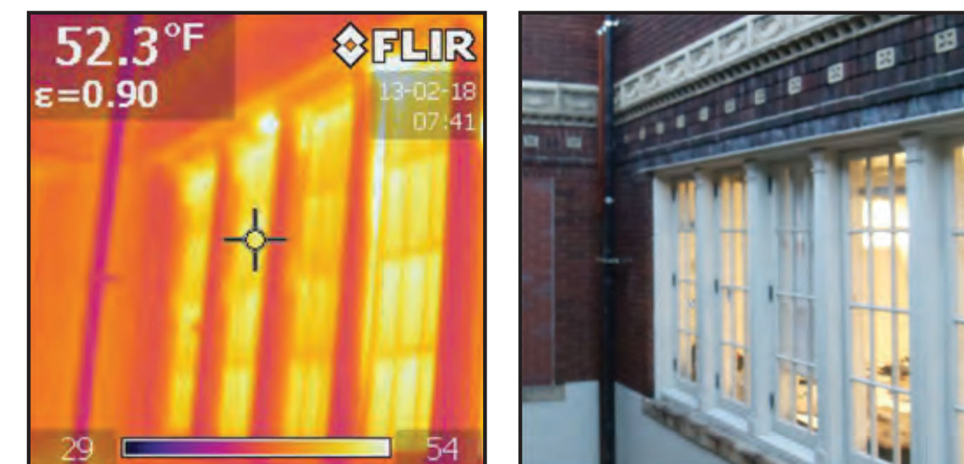
Figure 2.1 - Shattuck Hall pre-retrofit 1986. has an inefficient envelope, bridging a rate that keeps the exterior facade an average 15.5°F higher than the ambient outdoor air.
