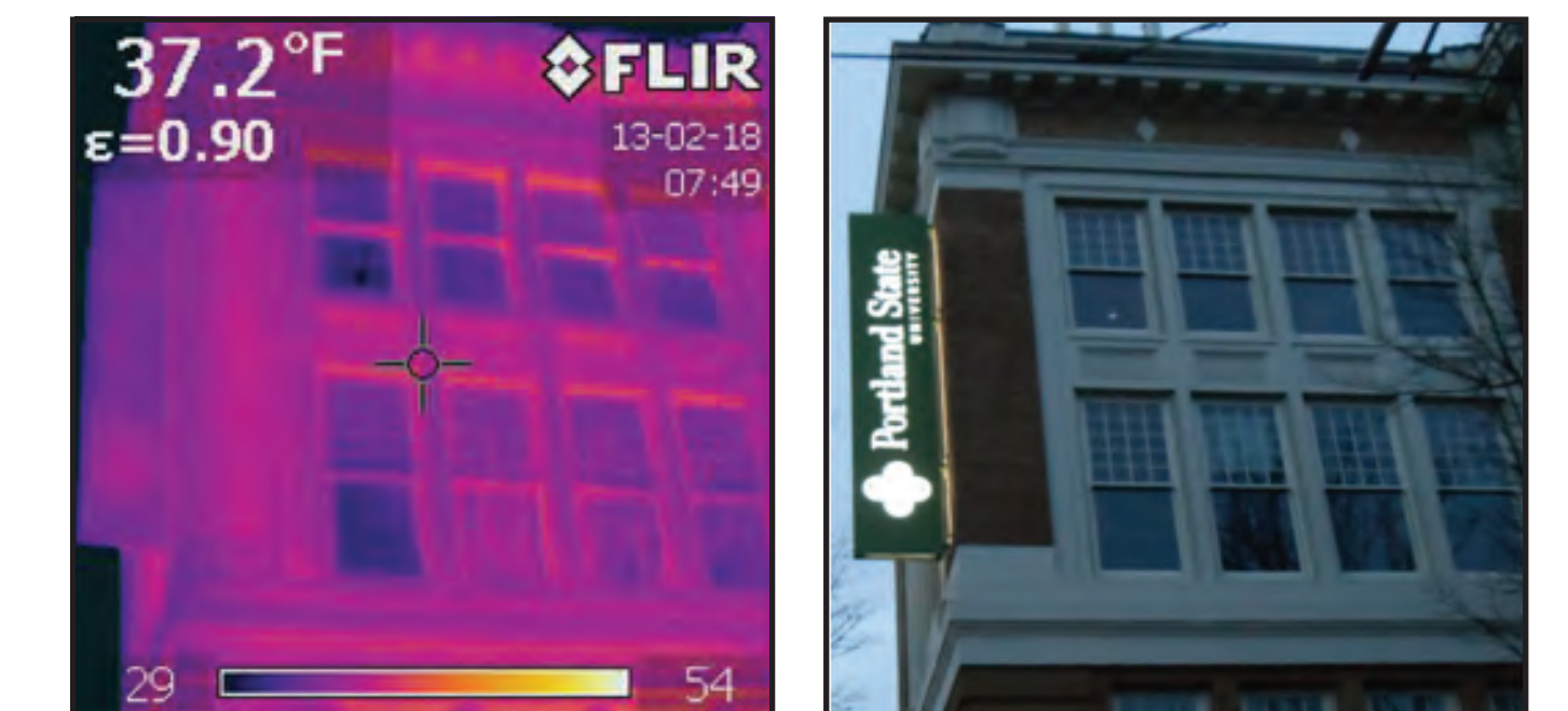
Figure 2.3 - Lincoln Hall post-retrofit 2010. has a highly efficient envelope, with a surface temperature equal to the ambient outdoor air.
