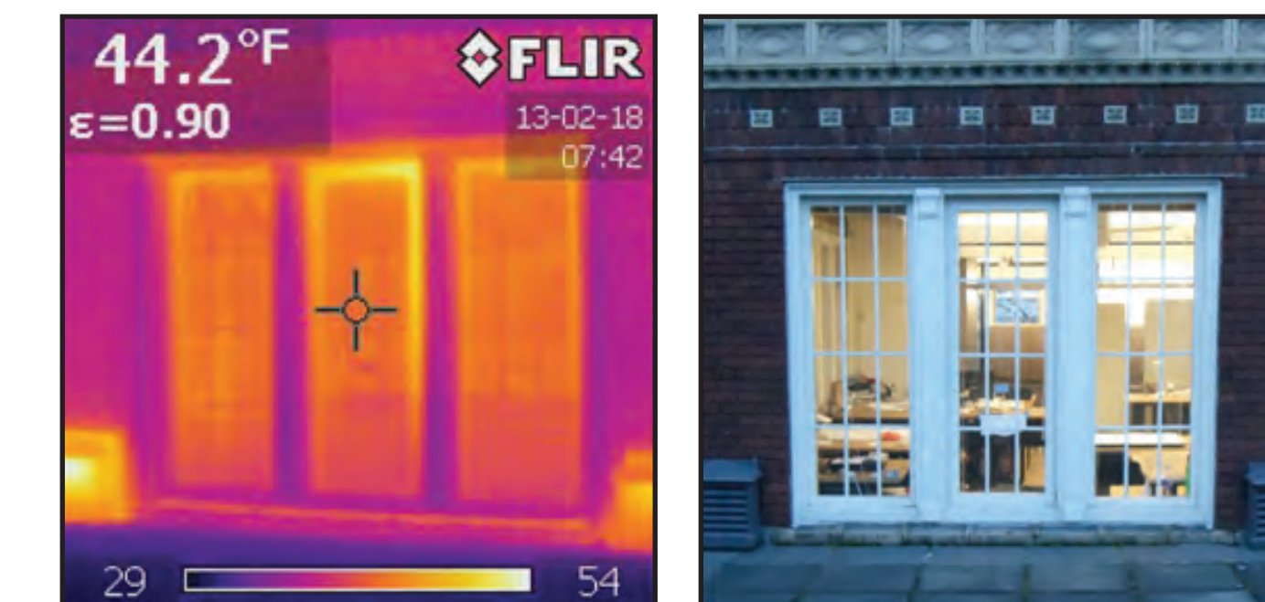
Figure 2.2 - Shattuck Hall post-retrofit 1986. has a leaky frame thermally bridging a rate that keeps the exterior facade an average 7.4°F higher than the ambient outdoor air.
