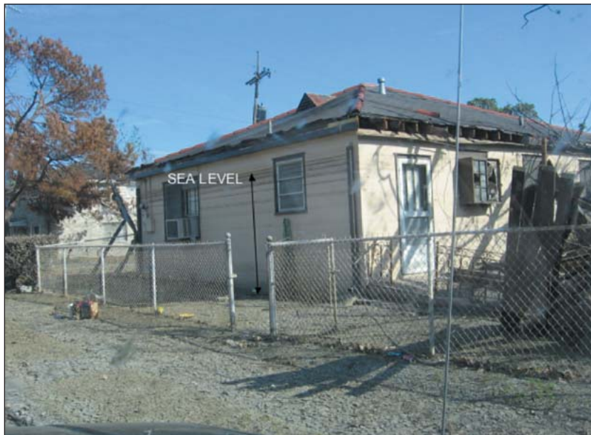
Figure 6. Photo of a house in the Lakeview area near the University of New Orleans, showing the depth of flooding in this area. After the levees broke, the water level was at sea level, showing the depth of subsidence due to soil oxidation after drainage of the organic wetland soils in this area.
