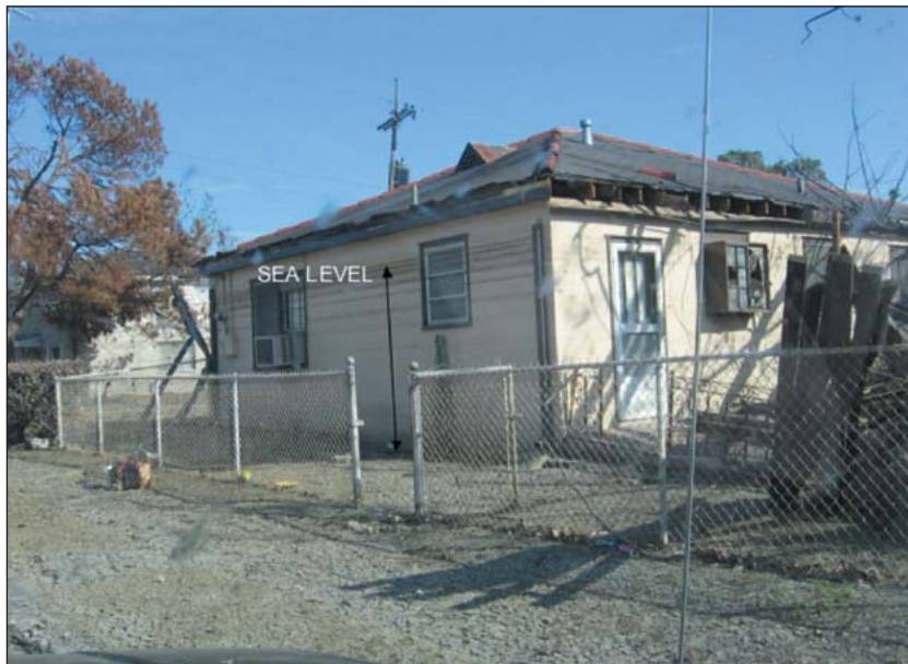
Figure 6. Photo of a house in the Lakeview area near the University of New Orleans, showing the depth of flooding in this area. After the levees broke, the water level was at sea level, showing the depth of subsidence due to soil oxidation after drainage of the organic wetland soils in this area.
