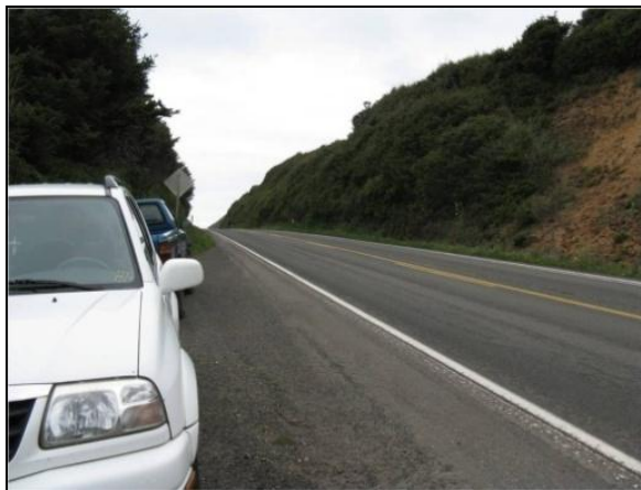
Figure 2. Road-cut area at Rock Creek – Big Creek Site, photo taken observing north from plot 8. Photo credit: Sara Zielin.
