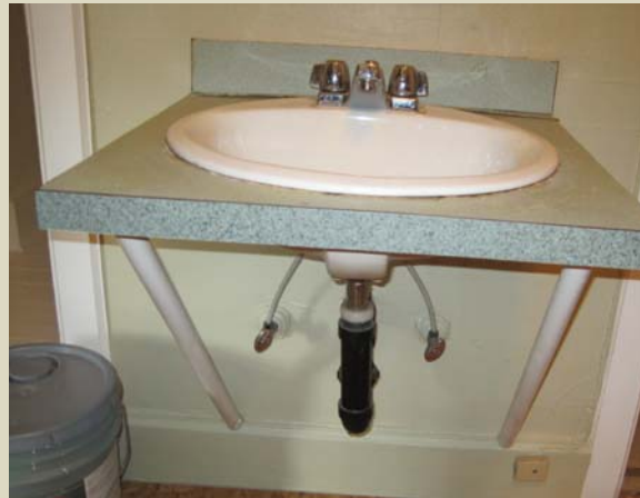
Sinks in units
