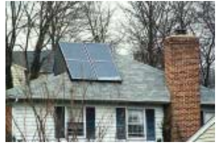
Solar panels serve as an alternative source of sustainable energy.
