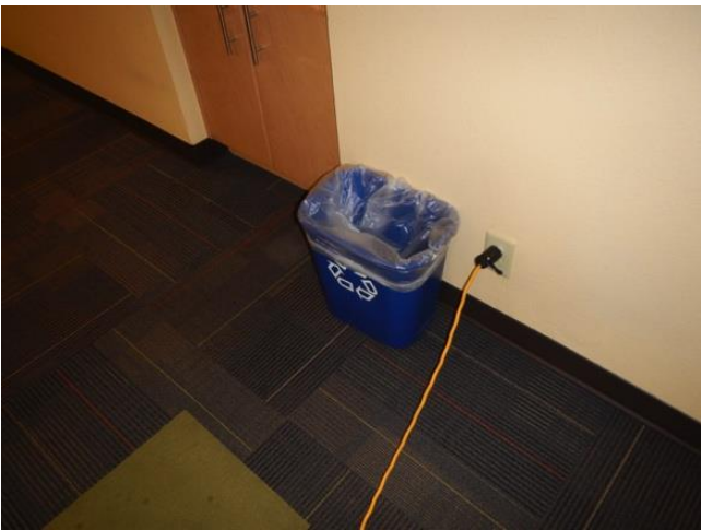
Image 3.1: Lone receptacle in hallway without clear signage
