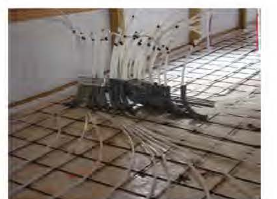
Radiant Heating and Cooling
