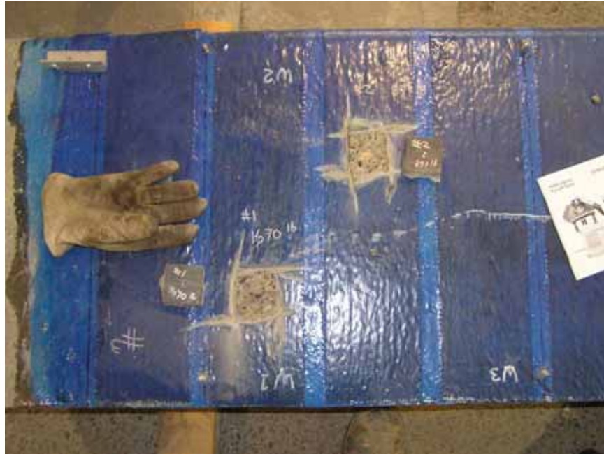
Figure B-4.4: Cohesive failure of concrete surface bonded to CFRP caused by direct-tension pull-off tests
