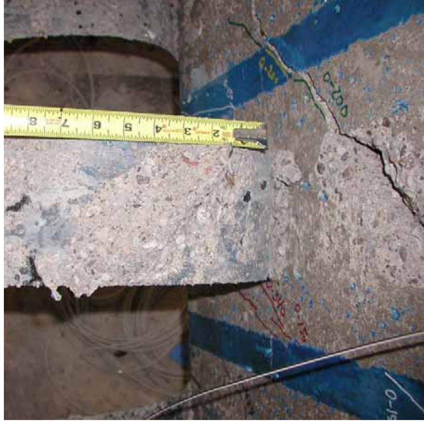
Figure B-5.7: Photograph of a debonded CFRP strip that formerly crossed a diagonal crack (post-failure of Specimen FC)
