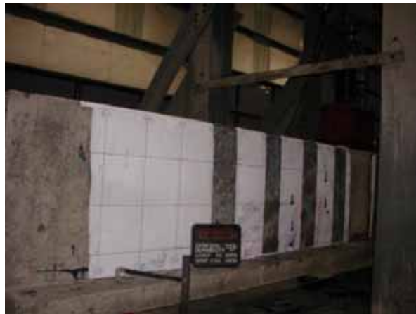
Figure 5.16: Failure photograph of Specimen IT12FTCK
