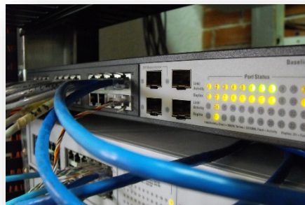
"Another Ethernet Switch in the Rack" by hdaniel is licensed under CC BY-SA 2.0
