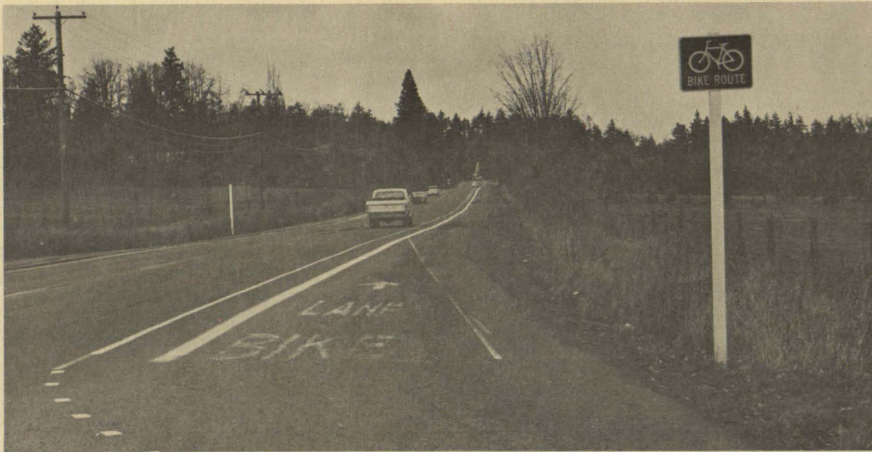
A Class III Bikeroute constructed on an extended shoulder and marked by signing and striping, located on State Highway 43 between Lake Oswego and West Linn, 1.8 miles long, cost $26,194 in 1973.
