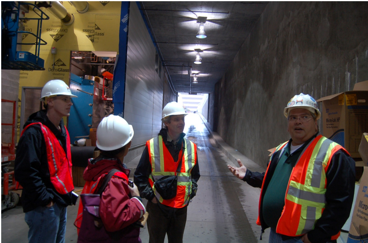
Adam Bonner, Site Supervisor for UO Arena/Hoffman Construction, leads MAK Court tour for designBridge Build/Tech class. Pictured here with Professor John Rowell and students.
