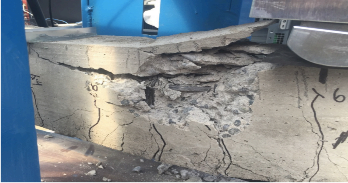
Figure 30: Crushing concrete cover
