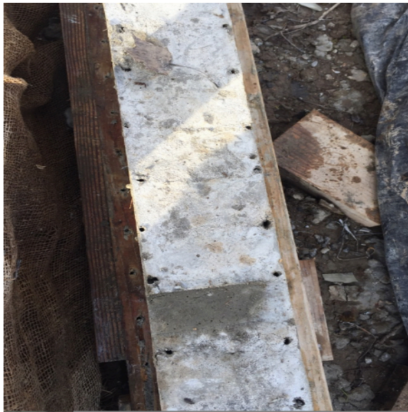
Figure 17: Voids representing deteriorated shear reinforcement
