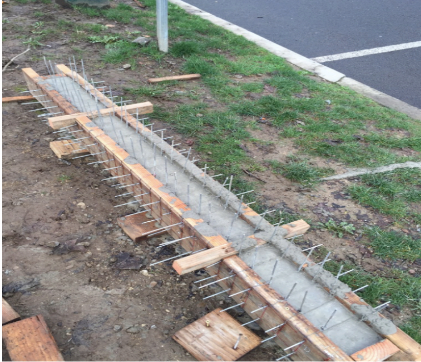
Figure 14: Temporary reinforcement in deteriorated Beam #4 &5
