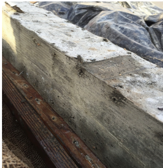
Figure 15: Shear voids in the deteriorated beam
