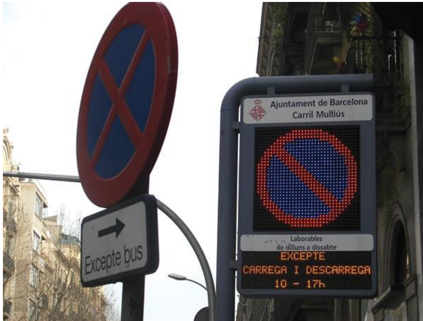
Figure 46. Variable message sign (VMS) displays
