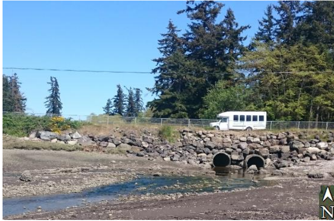
Figure 6: Erosion on the marine side of the Bucklin Hill Bridge culverts has created perched culverts above the stream bed thereby restricting access for incoming salmon to high tide periods. June 2015
