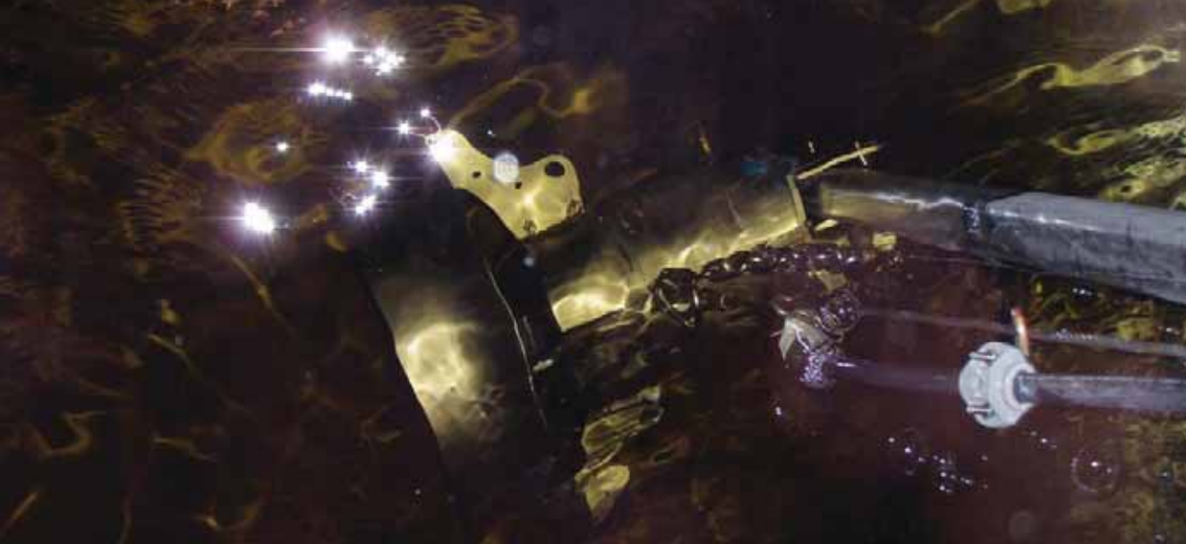
Treated wastewater to be reused within the La Center treatment plant.
