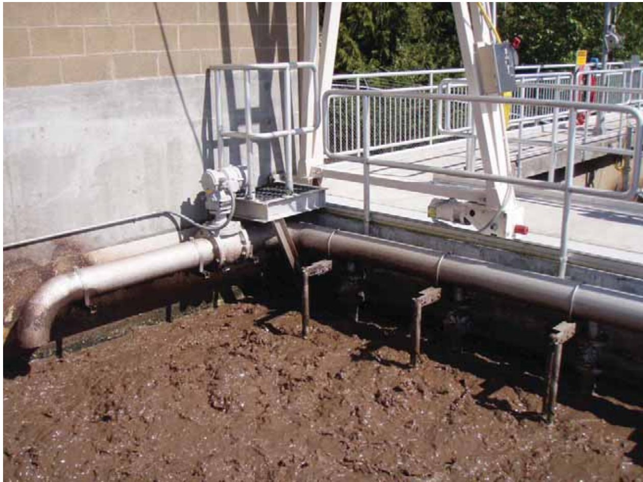
A tank at the small-scale municipal treatment plant in La Center, Washington.
