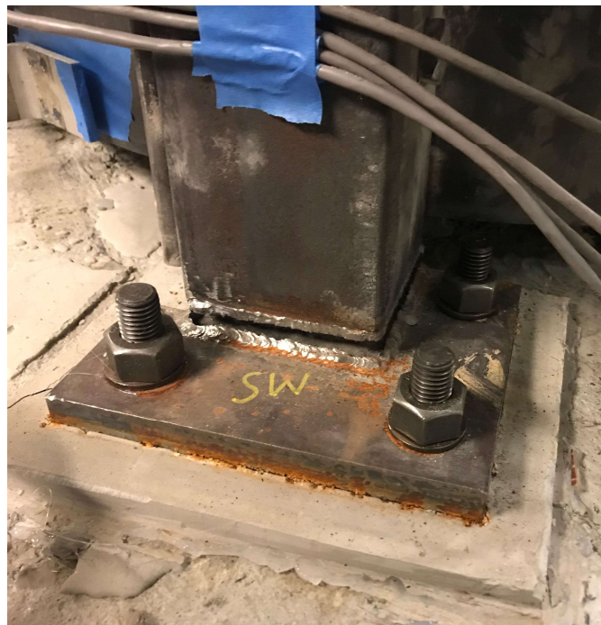
Figure 5.12: Hold-down weld failure
