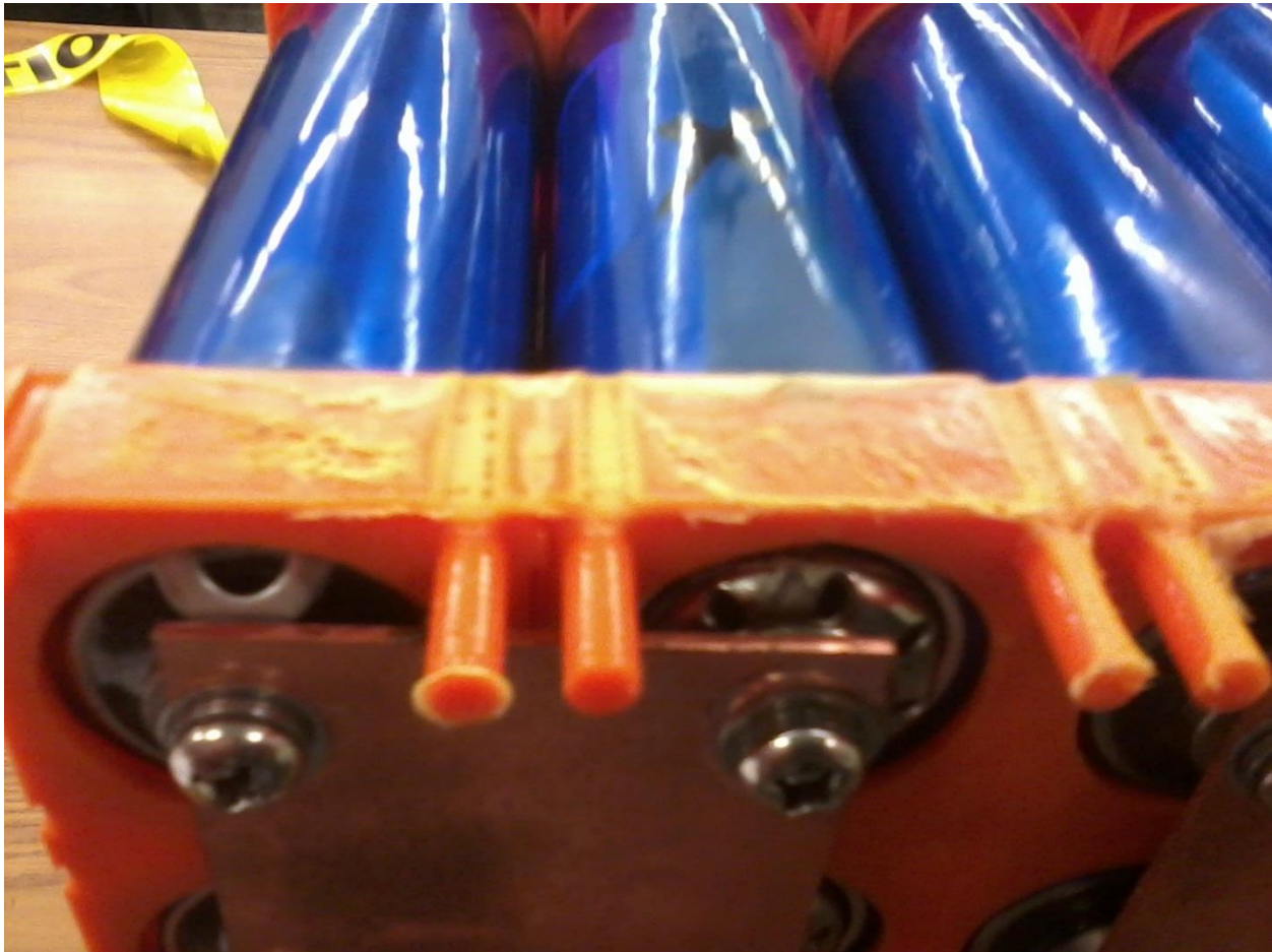
Figure 3.5 – The manufacturing defect discovered upon disassembly of one of the battery banks
