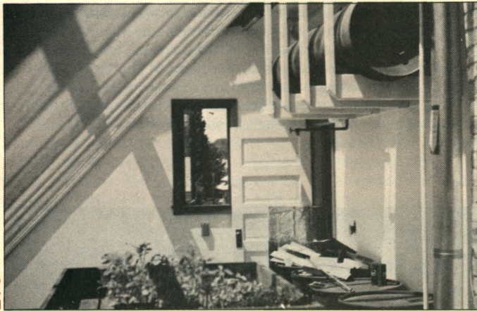
Water heater and plant starts in attic greenhouse at the Eliot Energy House.
