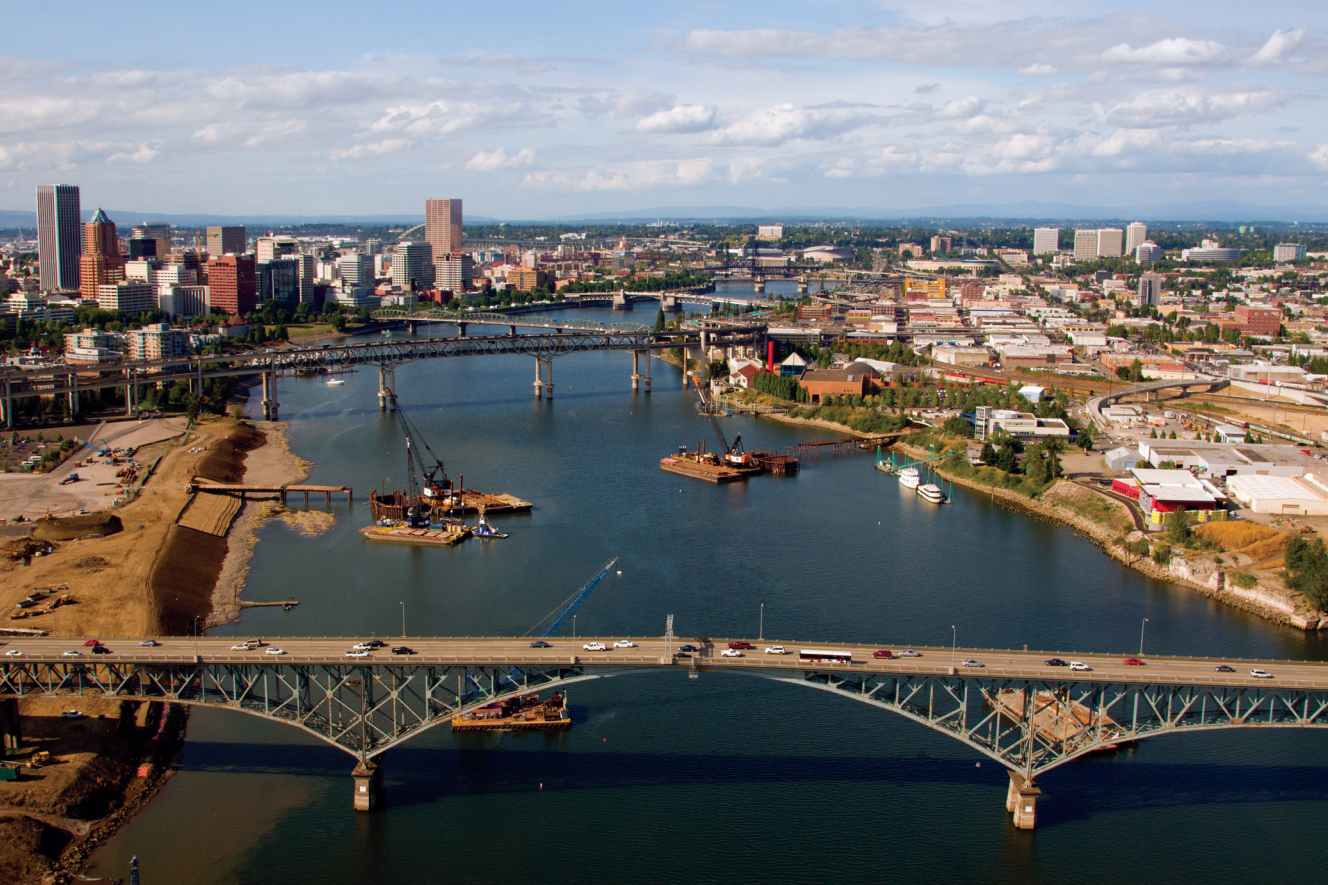
A view looking north from the Ross Island Bridge of TriMet's new transit bridge construction.
