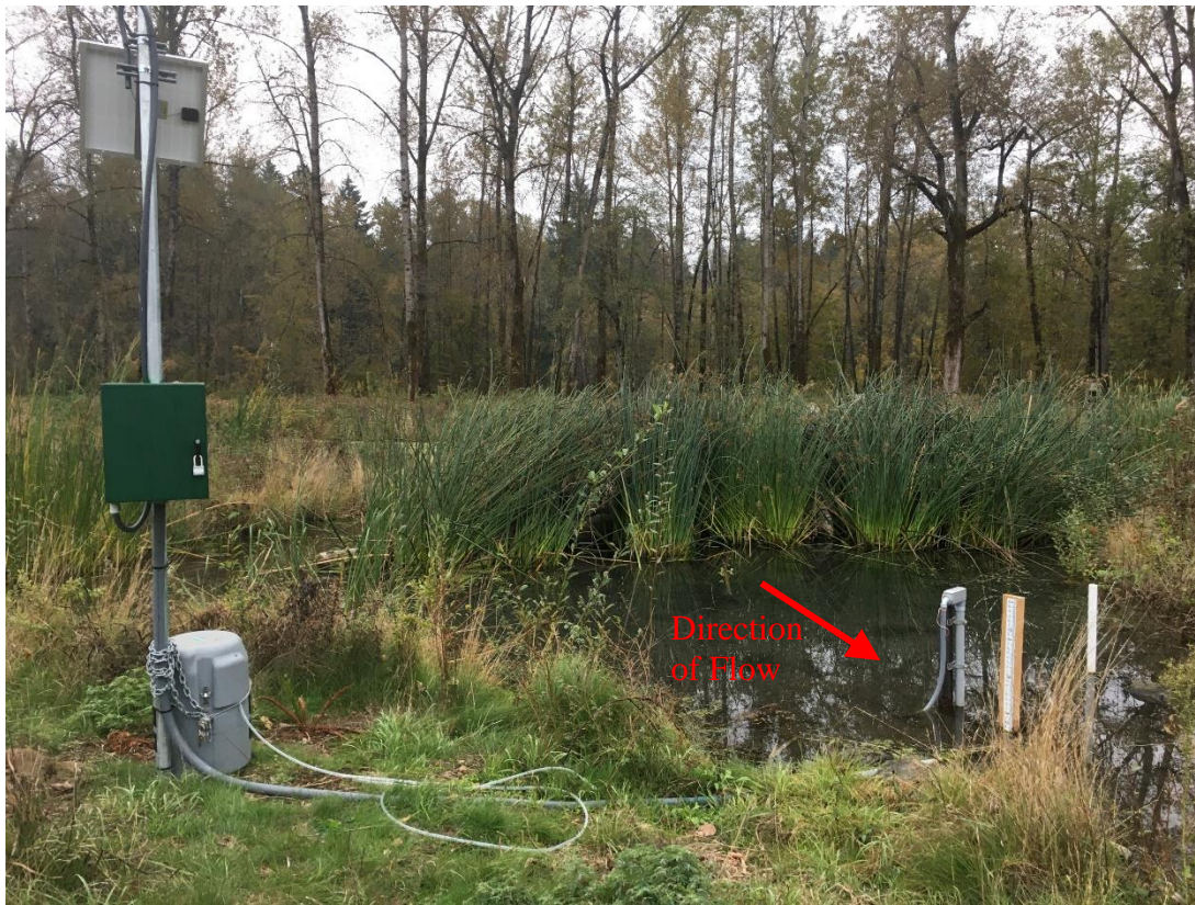
Figure 13. Portable autosampler being set-up at Monitoring Point 3.
