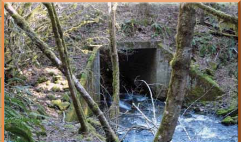
Williams Creek is an important travelway for aquatic and terrestrial wildlife, but the size and shape of the culvert, shown here, hindered passage for both. This culvert will be replaced during this STIP cycle, considering the needs of wildlife passage as well as aquatics. (Image: USDA Forest Service)
