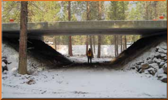
Shown while still under construction, the first wildlife underpass for the newly divided US 97 south of Bend will provide passage opportunities for all wildlife in the area when completed. This highway project incorporated many 'Green Highway' features, including wildlife crossing structures. (Image: Oregon DOT)
