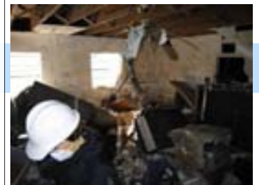
heavy flood damage
