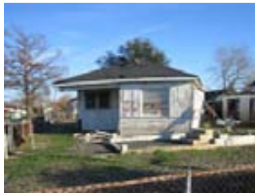
heavy structural damage
