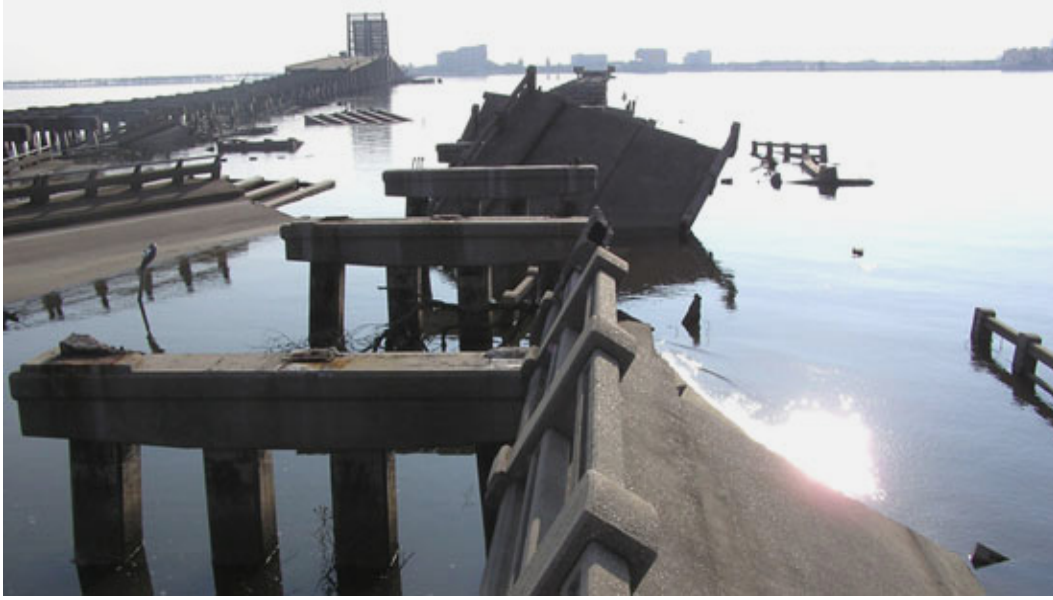
Figure 1.2. Damage to the U.S. 90 Biloxi Bay Bridge caused by Hurricane Katrina (courtesy of Solomon Yim, Oregon State University).
