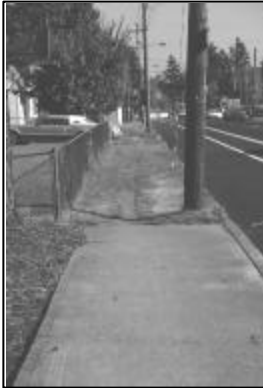
Gateway suffers from a sub-standard pedestrian environment
