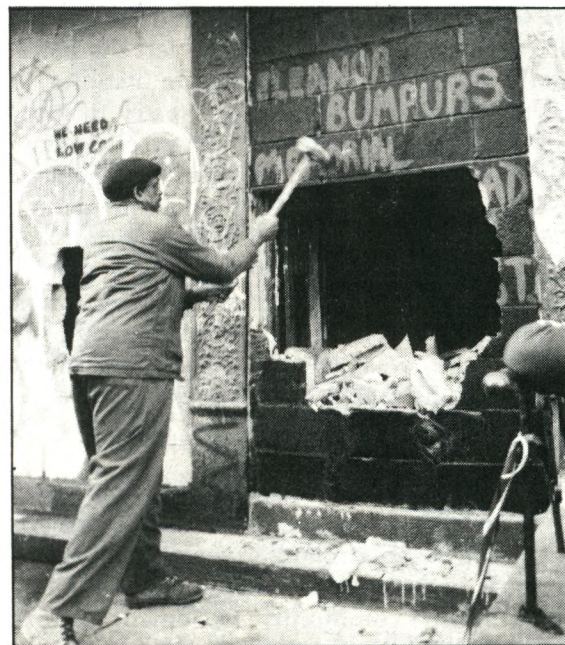
Homesteader takes turn at cinder block at housing project in New York's Lower East Side.
