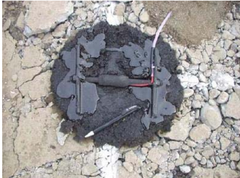
Figure 4: Close-up view of a strain gage over the rubblized JRC base course at the I-5 site.
