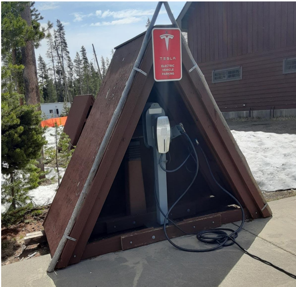
Figure 4. EV Charging Station at Crater Lake National Park (author's image).
