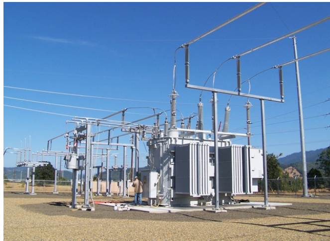
Figure 2.6: Author inspecting a 125 MVA 230-115 kV Load tap changing autotransformer
