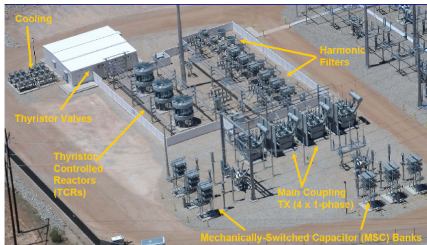
Figure 2.12: This SVC installation was in 2006 at St George Substation in Utah. The system voltage is 138 kV and the operating range is -35 to +100 MVar. [Sullivan and Hall, 2006]
