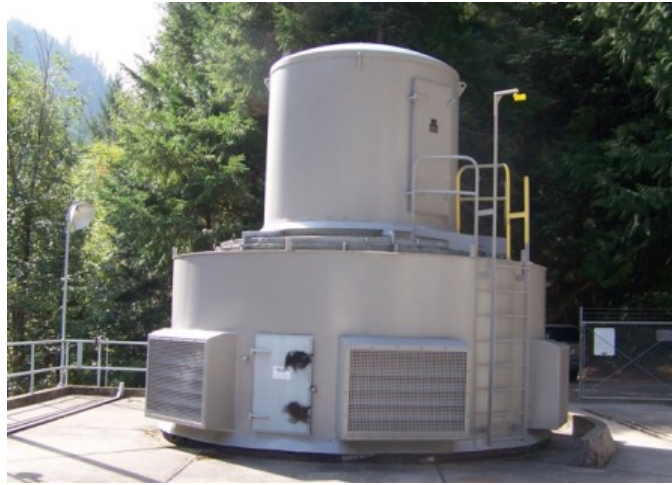
Figure 2.1: Picture of a 21 MVA hydro-electric generator
