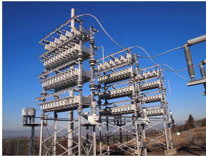
Figure 2.8: Example rack installation of a 50.4 MVar, 230 kV capacitor with 84 cans per phase. Note the reactor on the left for limiting inrush current.
