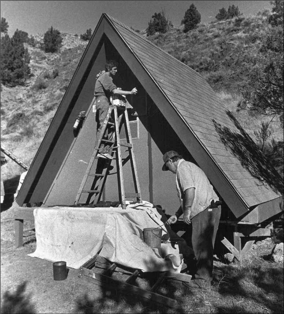
Two sannyasins paint and clean an A-frame structure built on old tent platforms for people experiencing homelessness. These structures were described by Rajneeshpuram as temporary housing, but state building officials disagreed because they were heated and wired for electricity.
