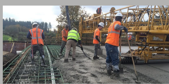
Placing the deck for the new Fifth Plain Creek Bridge. Source: Clark County
