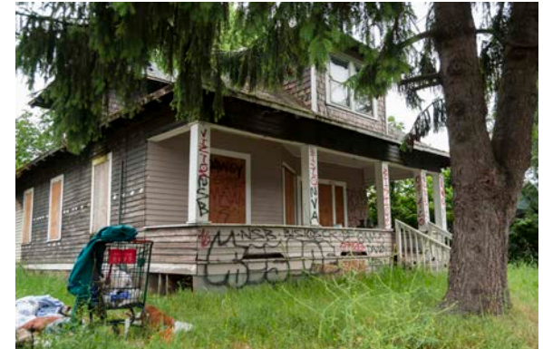
(above) An abandoned home, called a “zombie house” by neighbors, on SE Reedway St.
