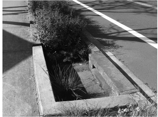
Figure 8. Bioswale inlets in the USA
