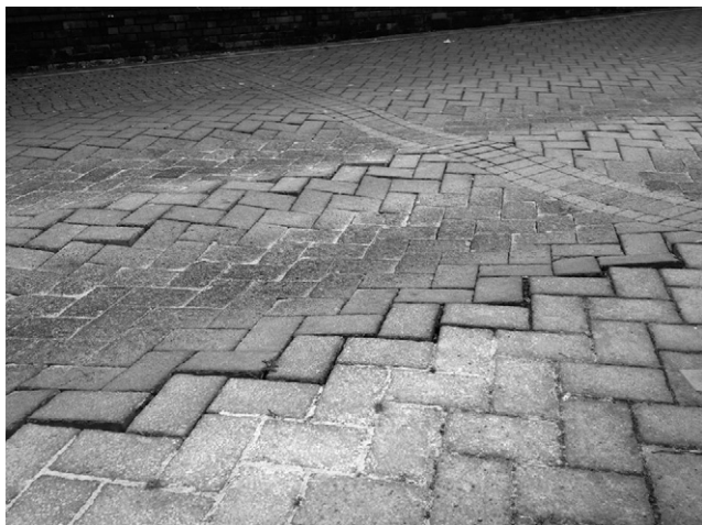
Figure 10. Sunk paving at UK site
