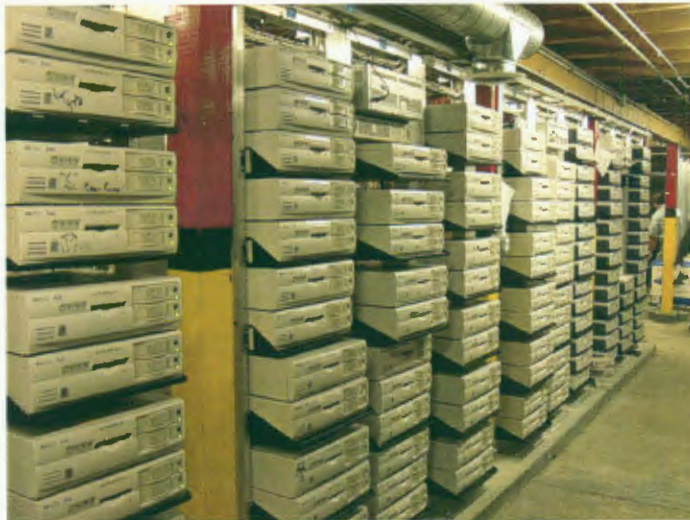
Typical data center, housing Internet servers
