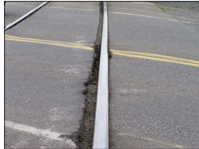
An undesirable railroad crossing condition for bicyclists
