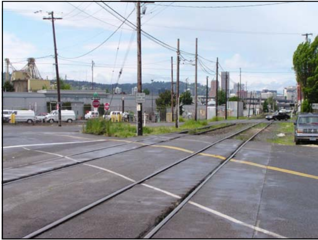
An undesirable railroad crossing condition for bicyclists
