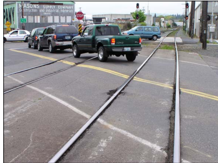
The railroad track crossing on SE Clinton at SE 11th and SE 12th is undesirable due to the wide flange, pavement cracking, and a 38° angle track crossing.
