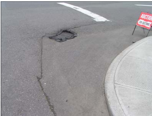
A drainage gate indicates where the old curb was before a new curb was installed to make turning large trucks easier. The new curb lacks an ADA required ramp.
