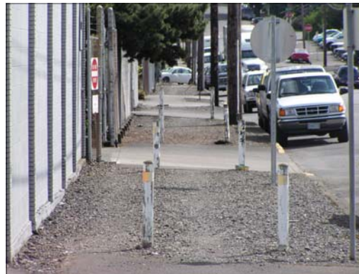
Demand paths indicate where a sidewalk should be. Instead, the pavement is intermittent, located only at the driveways.
