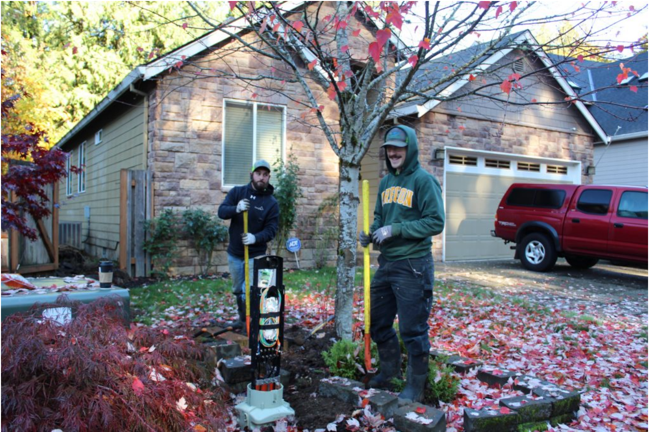
SandNet utility workers Chris Krieger and Peter Light install a new connection for a residential customer
