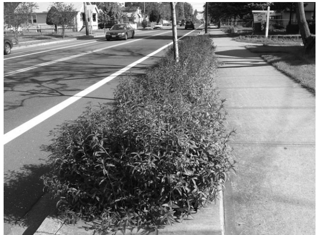
Figure 4 Bioswale not extending into the road.
