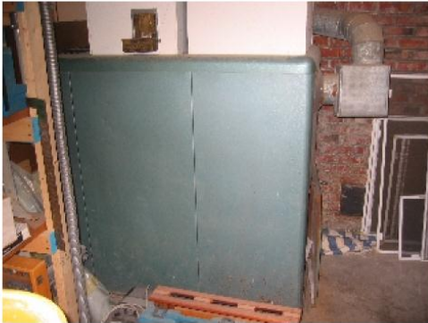
Oil converted to gas furnace.
