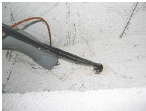
Air leakage through holes in basement rim joist.
