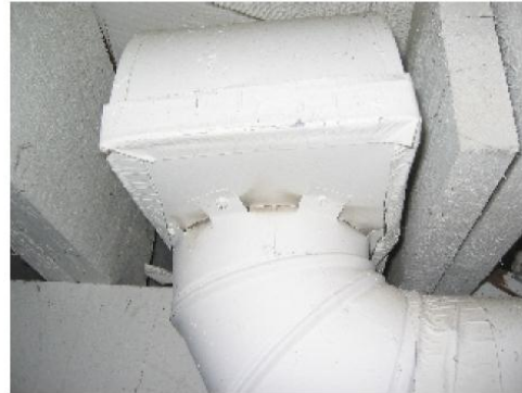
Leaky tabbed connection.
