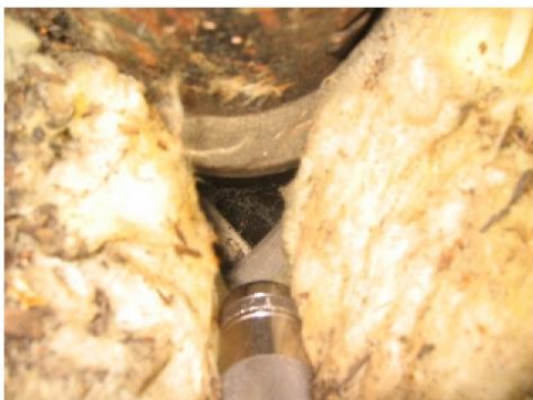
Air leakage at main plumbing stack in attic.
