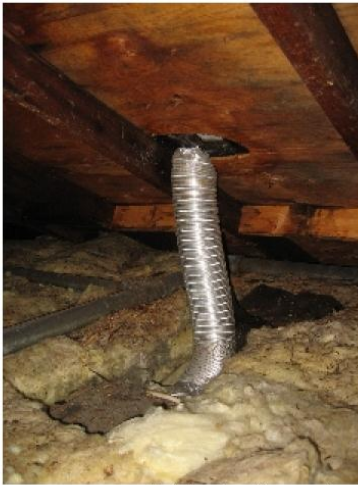
Bath fan ducted improperly to roof vent.
