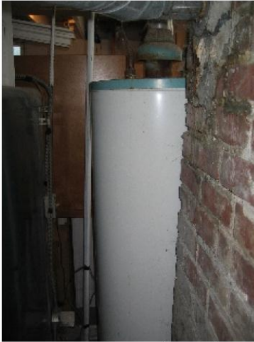
Gas water heater.
