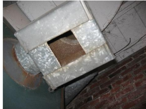
Furnace draft hood: exhaust gases inside.
