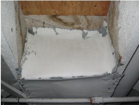
Leaky panned joist duct.
