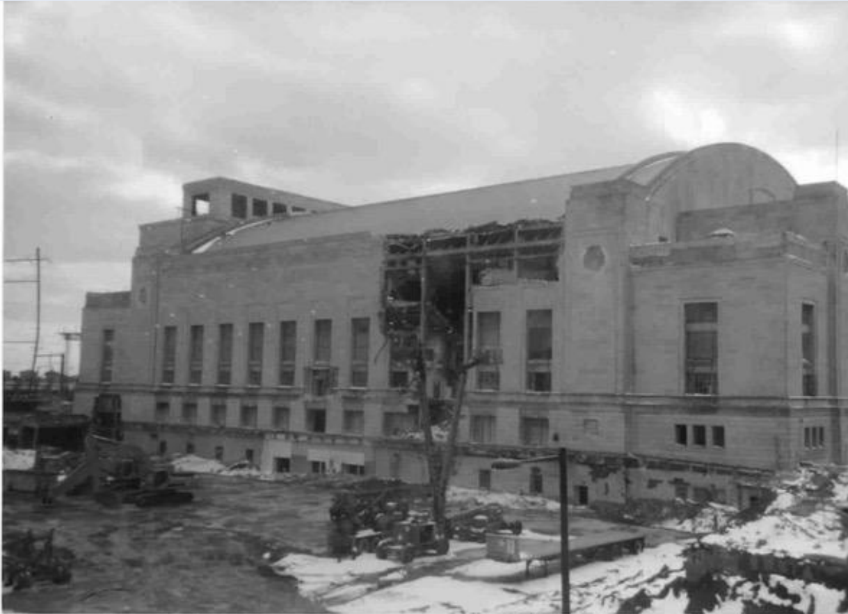
FIGURE 7.5 Philadelphia Convention Hall and Civic Center at beginning of demolition in 2005. Credit: William Keller.
