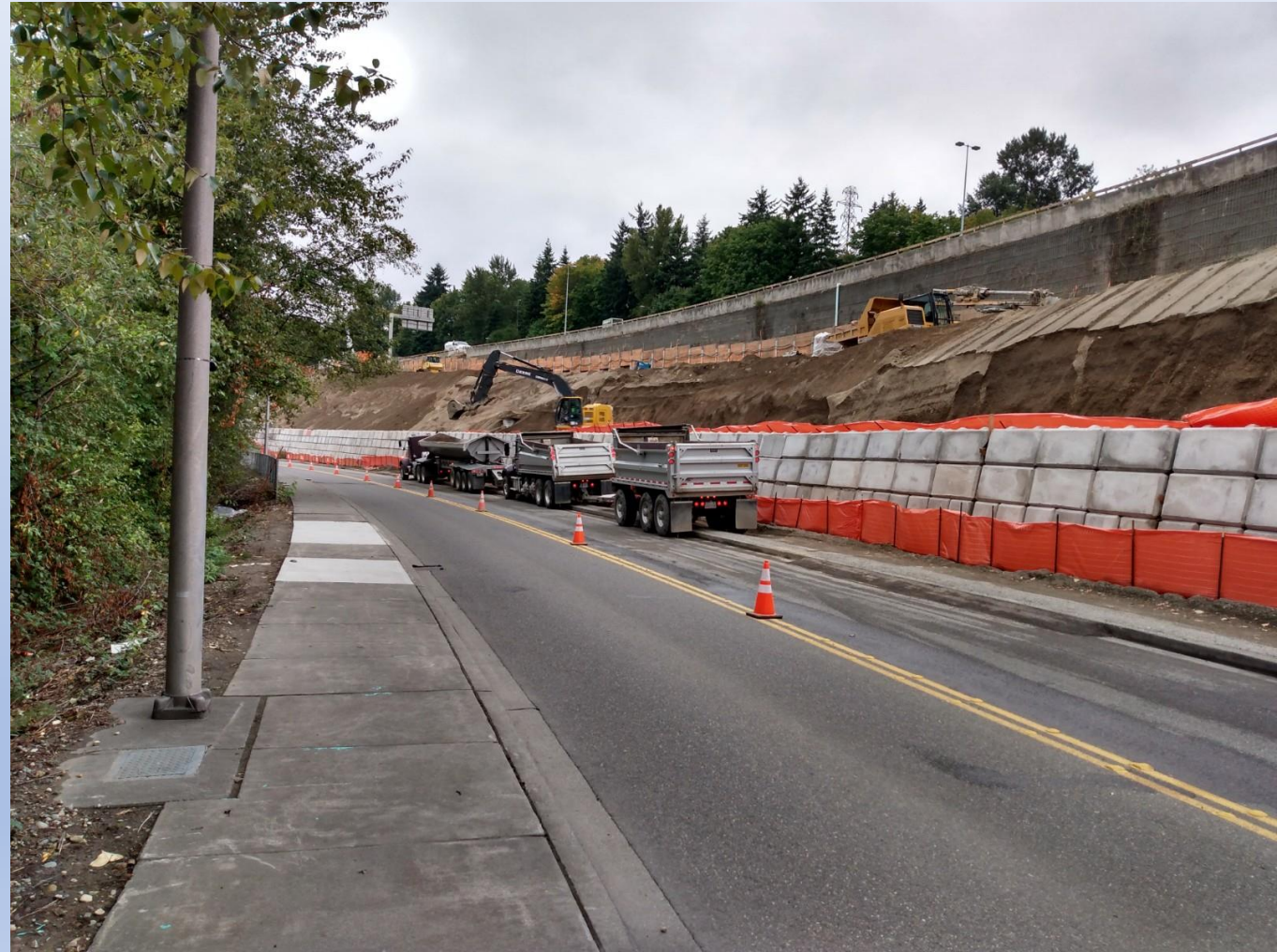
I 405 being widened in Renton just now. Bellevue LRT opening postponed again.
