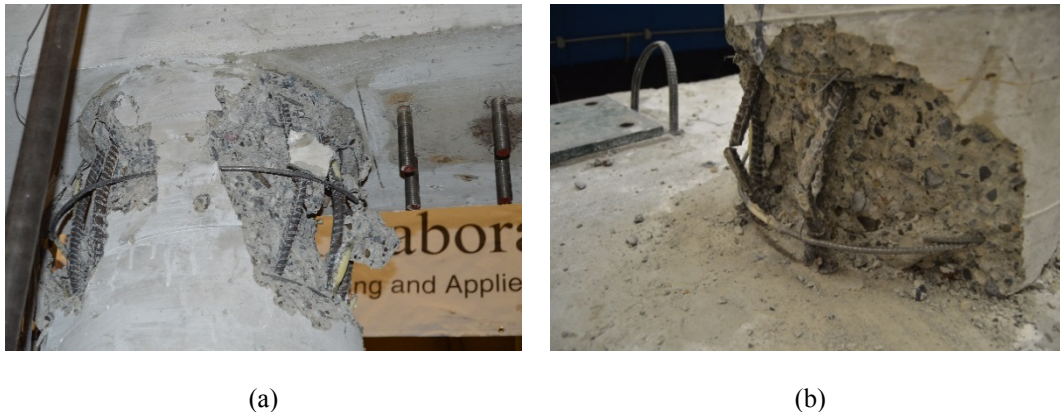
Figure 7.23: Damage on As-built RC bent. (a) Buckling of Steel, (b) Rupture of steel
