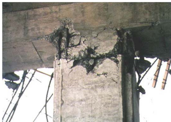
Figure 5.1: Poorly Confined Column in 1971 San Fernando Earthquake
