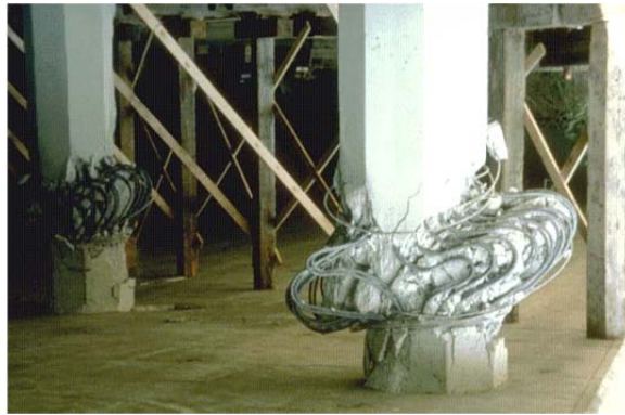
Figure 5.3: Damage in RC columns on the Simi Valley Freeway during the 1994 Northridge Earthquake ( Teng 1994 )
