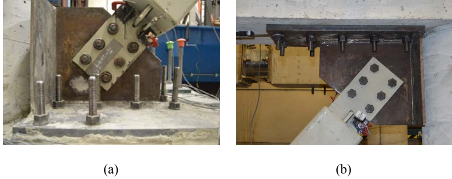
Figure 7.7: No Gusset Plate to Column Connection (a) Lower connection, (b) Top connection
