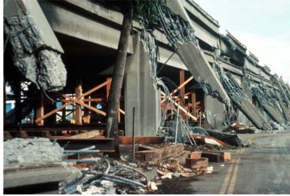
Figure 5.2: Collapsed Cypress street viaduct in Oakland during the 1989 Loma Prieta Earthquake ( USGS and Wilshire 1989 )
