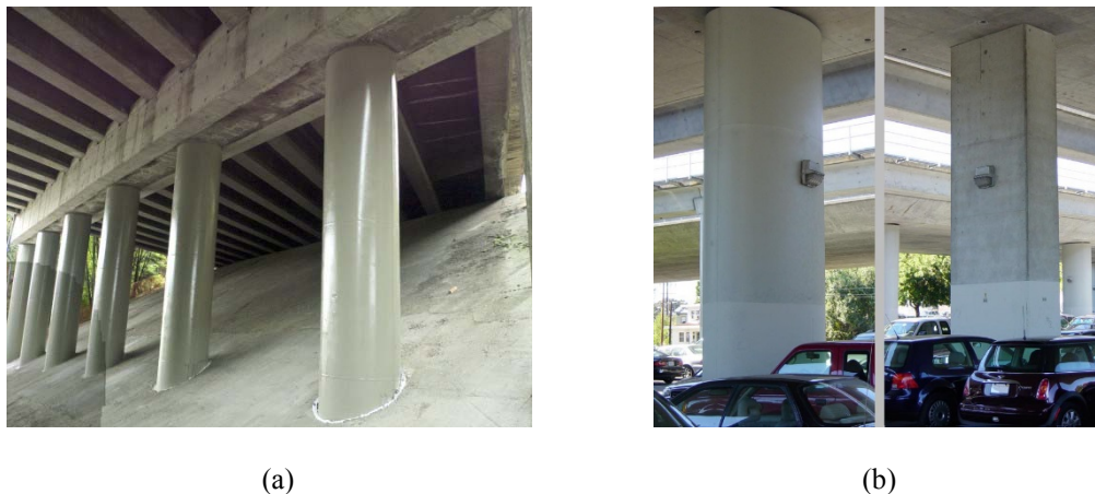
Figure 5.8: Steel Jacketing for; (a) circular columns in bridge along Interstate 5, Seattle (photo: Lucia Bill), (b) rectangular column in bridge State Route 24 eastbound, San Francisco. Left: retrofitted column. Right: As-built column (photo, Leonard G.)
