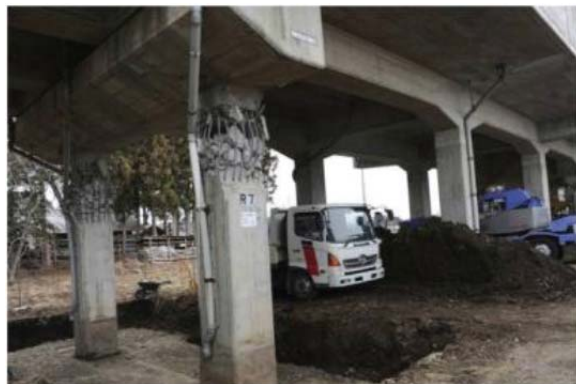
Figure 5.4: Damage in Nakasone viaduct during 2011 Japan earthquake ( Kawashima et al. 2011 )
