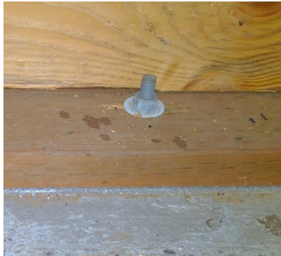
A home that is not properly bolted to its foundation could slide off of it during a CSZ earthquake, making it unsafe for occupation
