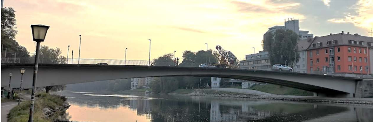
Figure 3: Photo of Gänstorbrücke, built 1950, prestressed concrete, over the river Danube from Ulm to Neu-Ulm. Some tendon wires suffer from 50% cross section loss due to corrosion [2].
