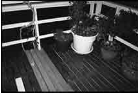
Figure 67: Repairs to My Deck: I like to try and keep up on house repairs.
