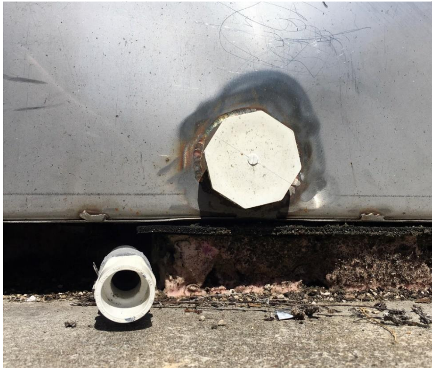
Figure 4. Closeup of outflow pipe and one closed overflow pipe.
