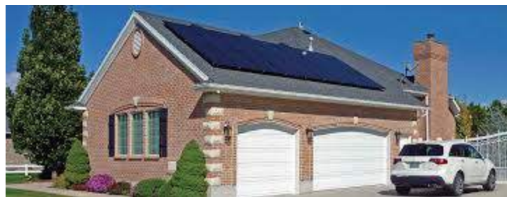
Figure 7: Asphalt Shingle with Solar Panel System
