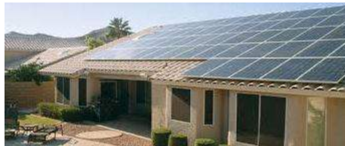
Figure 6: Ceramic Tiles with Solar Panel System
