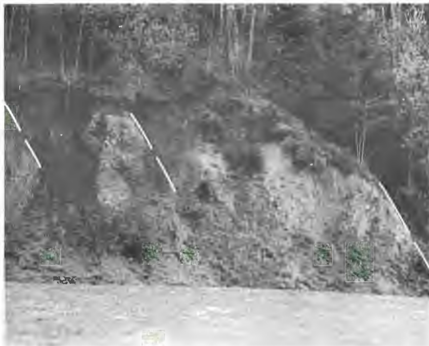
Figure 8. Part of a wide, west-trending, zone of normal faulting in a road cut on S.W. Terwilliger Boulevard. Note the three distinct fault planes separating highly fractured and weathered basalt.
