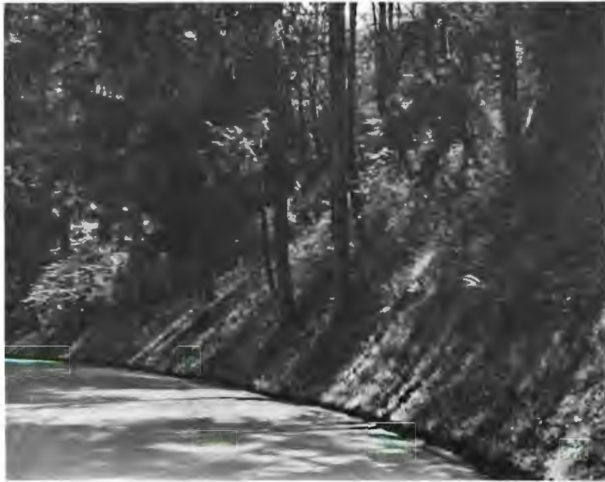
Figure 4. Photo of potentially unstable site; bent tree trunks indicate area of soil creep.
