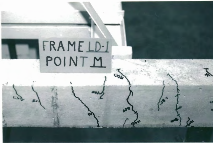
Fig. 5.27. Flexural cracks near M
