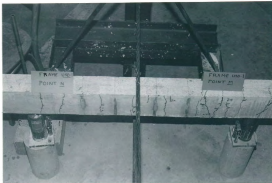
Fig. 5.14. Flexural cracks in the middle third of the beam
