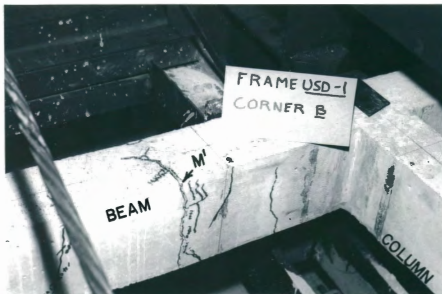
Fig. 5.16. Flexural-shear crack at M' (positive moment cutoff point)
