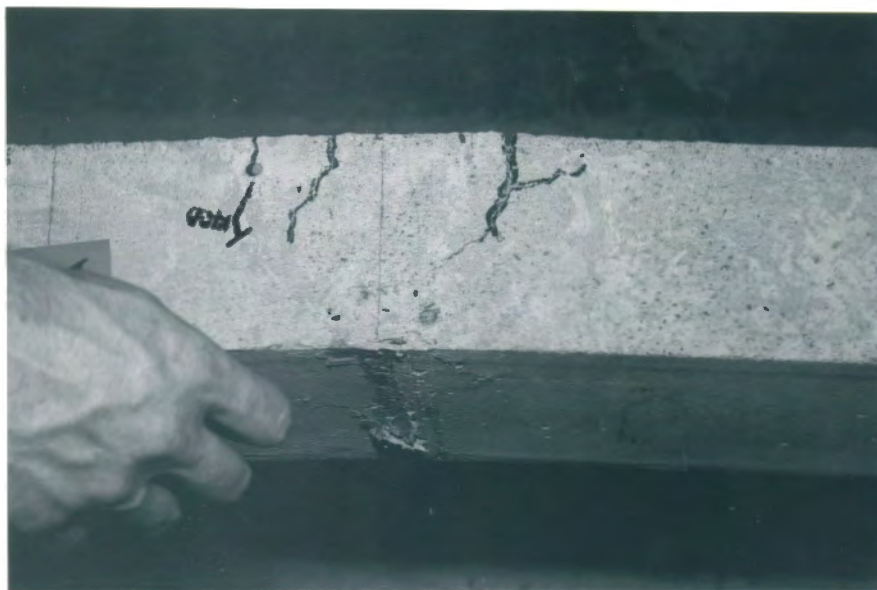
Fig. 5.26. Flexural-shear crack at negative moment cutoff point
