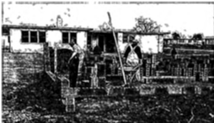
Figure 3-8. (photo) Construction of modernist housing of Jersey Homesteads, a utopian experiment, Hightstown, NJ, November 1936. The community is now part of Roosevelt, NJ. Architects retained were Louis J. Kahn and Alfred Kastner. Photographer Russell Lee. Courtesy Library of Congress Prints & Photographs Division, FSA-OWI Collection (LC-USF33-011030-M5 DLC).
