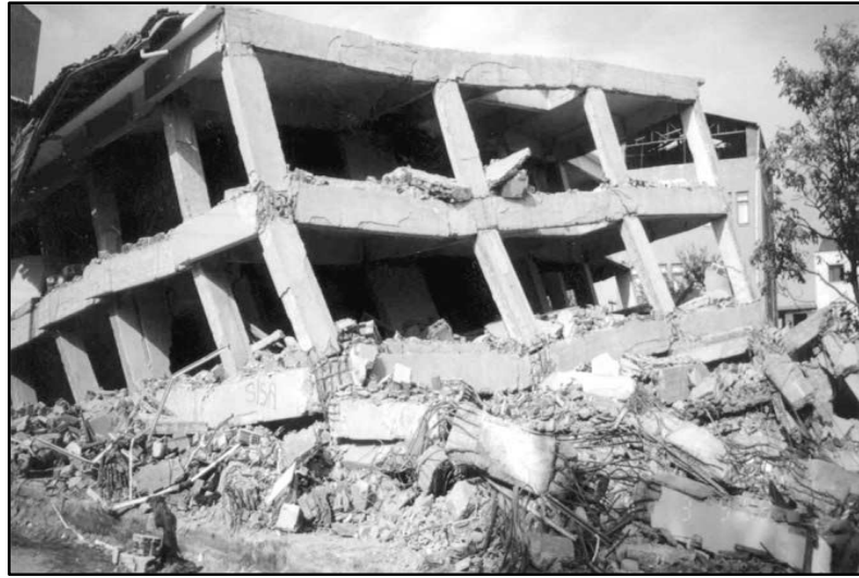
Figure 1-1 Beam-Column Joint Shear Failure, Kocaeli Earthquake
