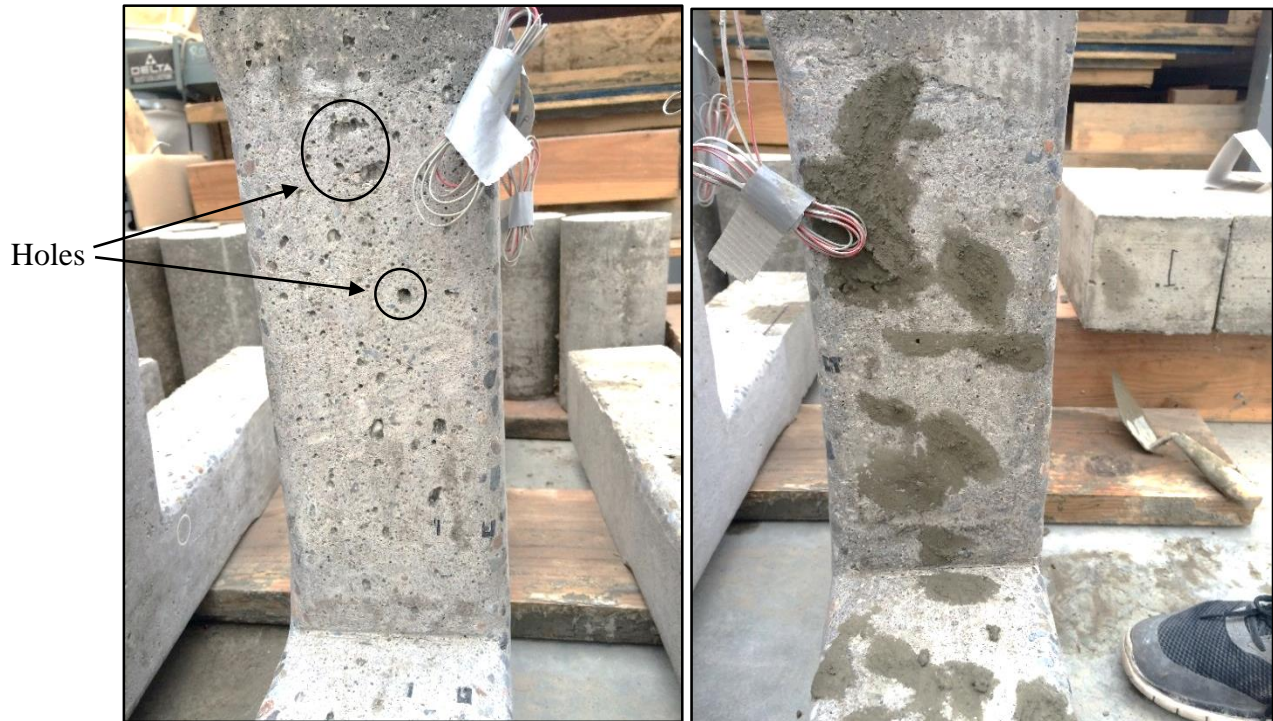
Figure 3-22 Holes on the Concrete Surface
