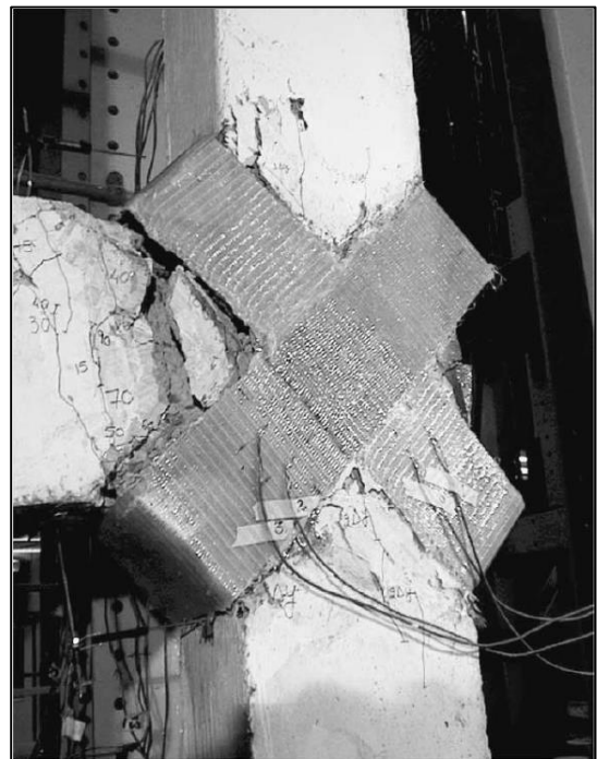
Failure Mode of Joint T9
