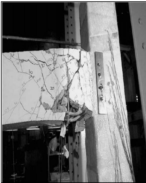
Failure Mode of Joint T2R
