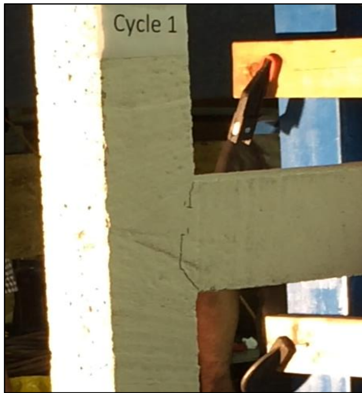
Figure 4-12 The Cracks of Joint J2 at the End of Cycle 1
