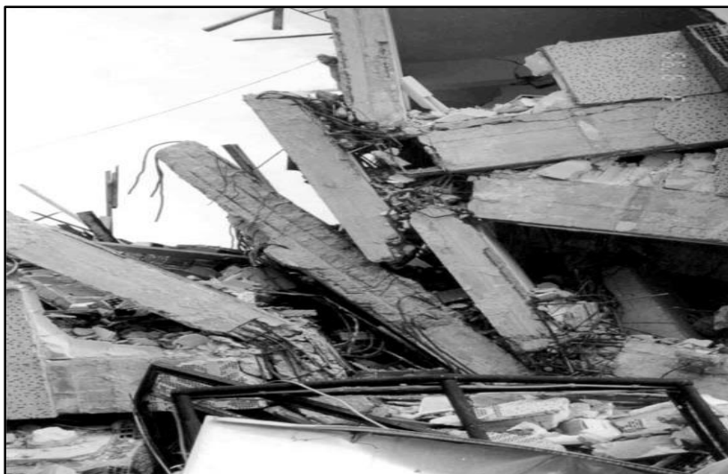
Figure 1-2 Joint Failure, Kocaeli Earthquake
